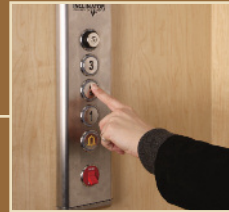
Cab Operating Panel, with remote call stations at each landing's door.
